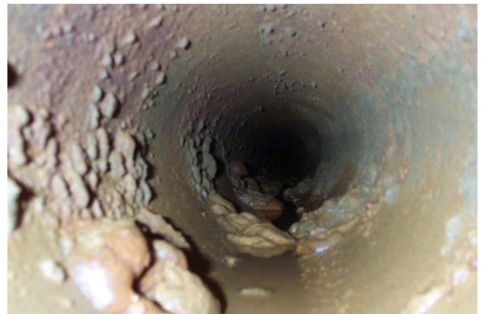
Tuberculation in sprinkler pipe caused by microbial activity.
