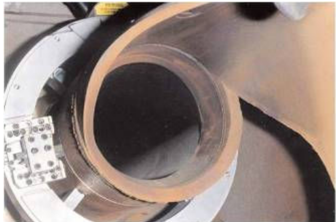
A rupture of a feedwater line at a coal-fired plant was caused by erosion/corrosion-induced wall thinning.
